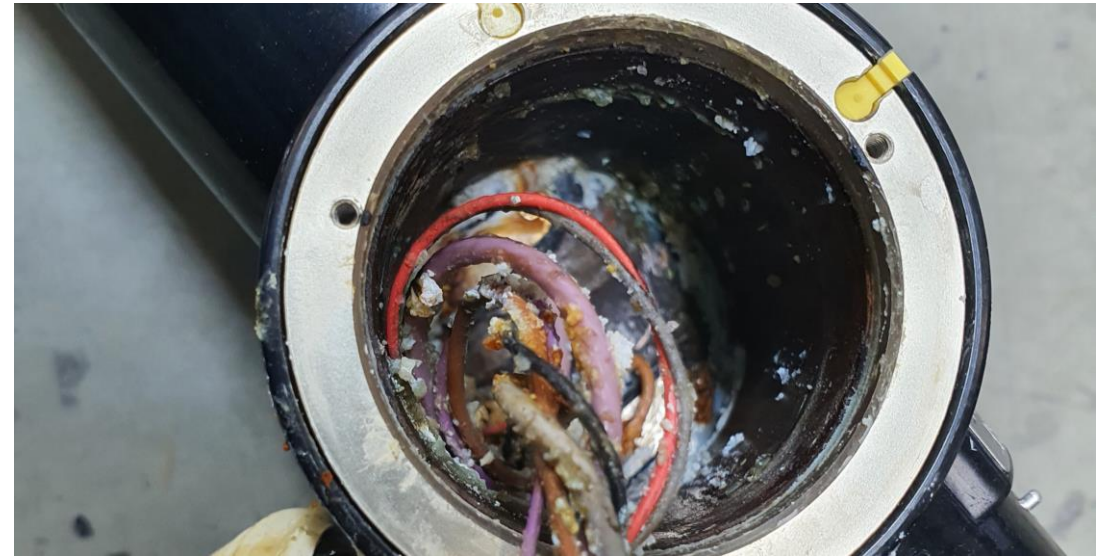
Moisture penetration in the supply plug
